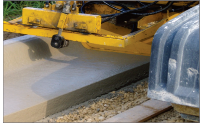
Curb machine radius with no tears in the concrete.
